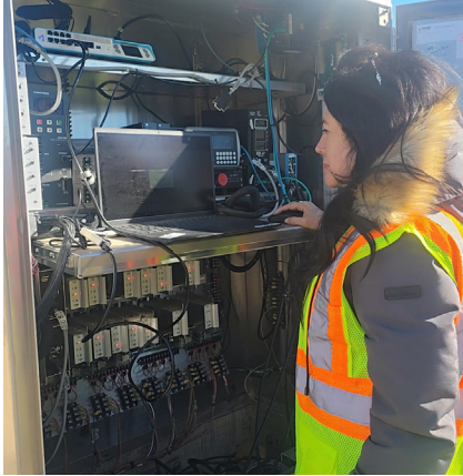
Alarcon working on software in a traffic control cabinet.
