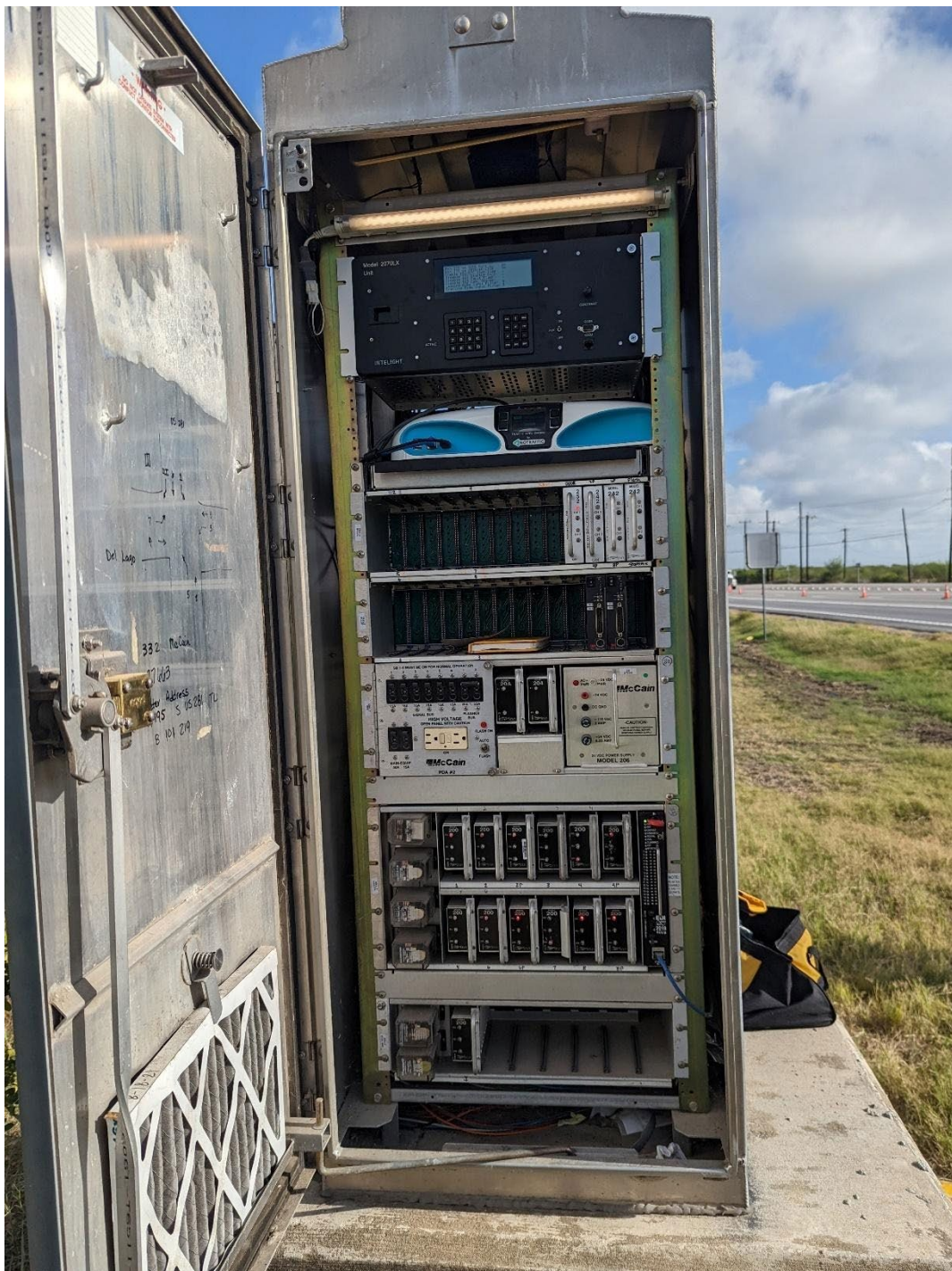
Figure 7: Front view of 332 cabinet after installation.
