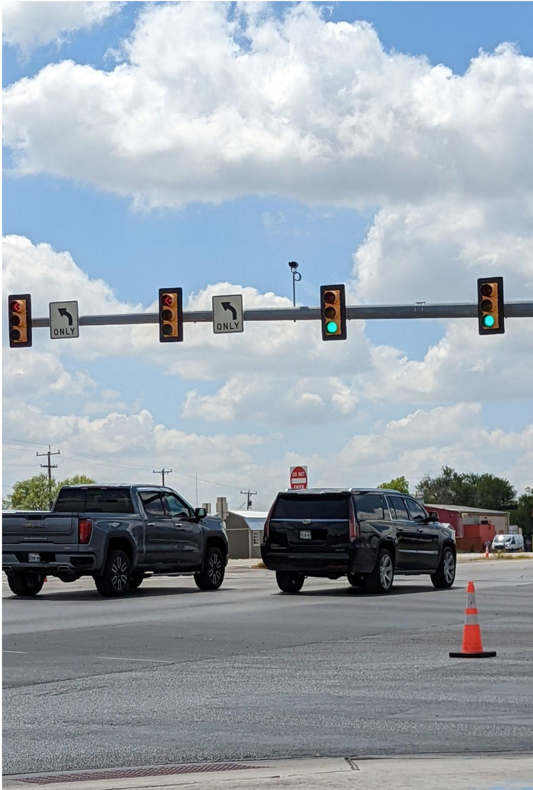
Figure 11: Sensor unit installed at one approach
